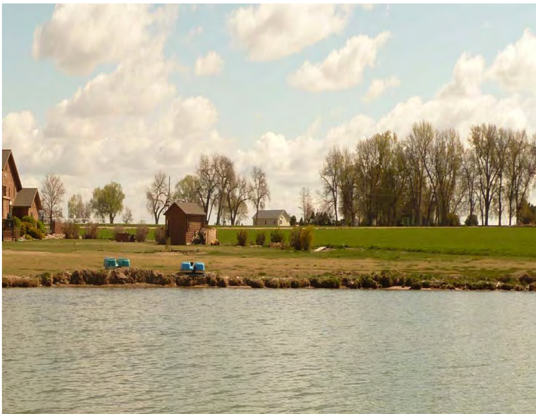
Photo 12. May 2, 2011. Looking north, northeast at wave action and resulting erosion along northern shoreline. Here there is no wetland vegetation edge to buffer the shoreline.
